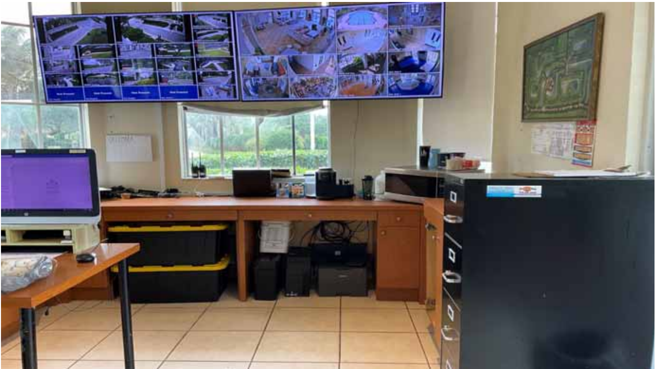
Gatehouse Security Cameras
