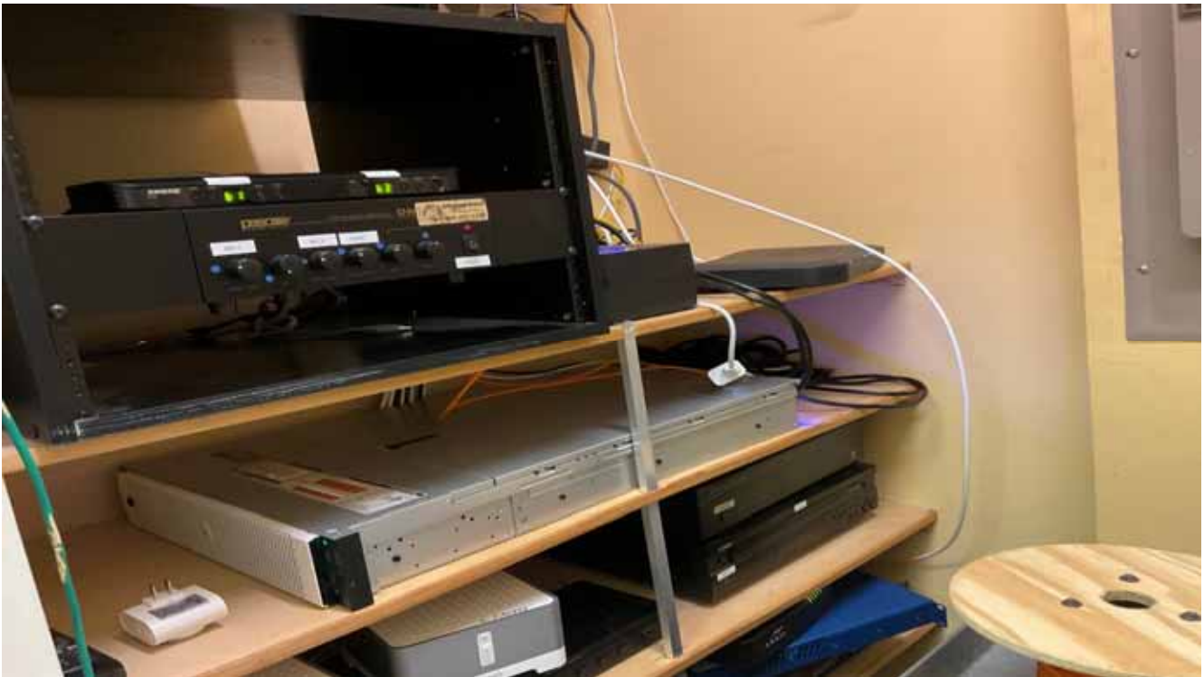
Clubhouse - Sound System & WIFI Equipment
