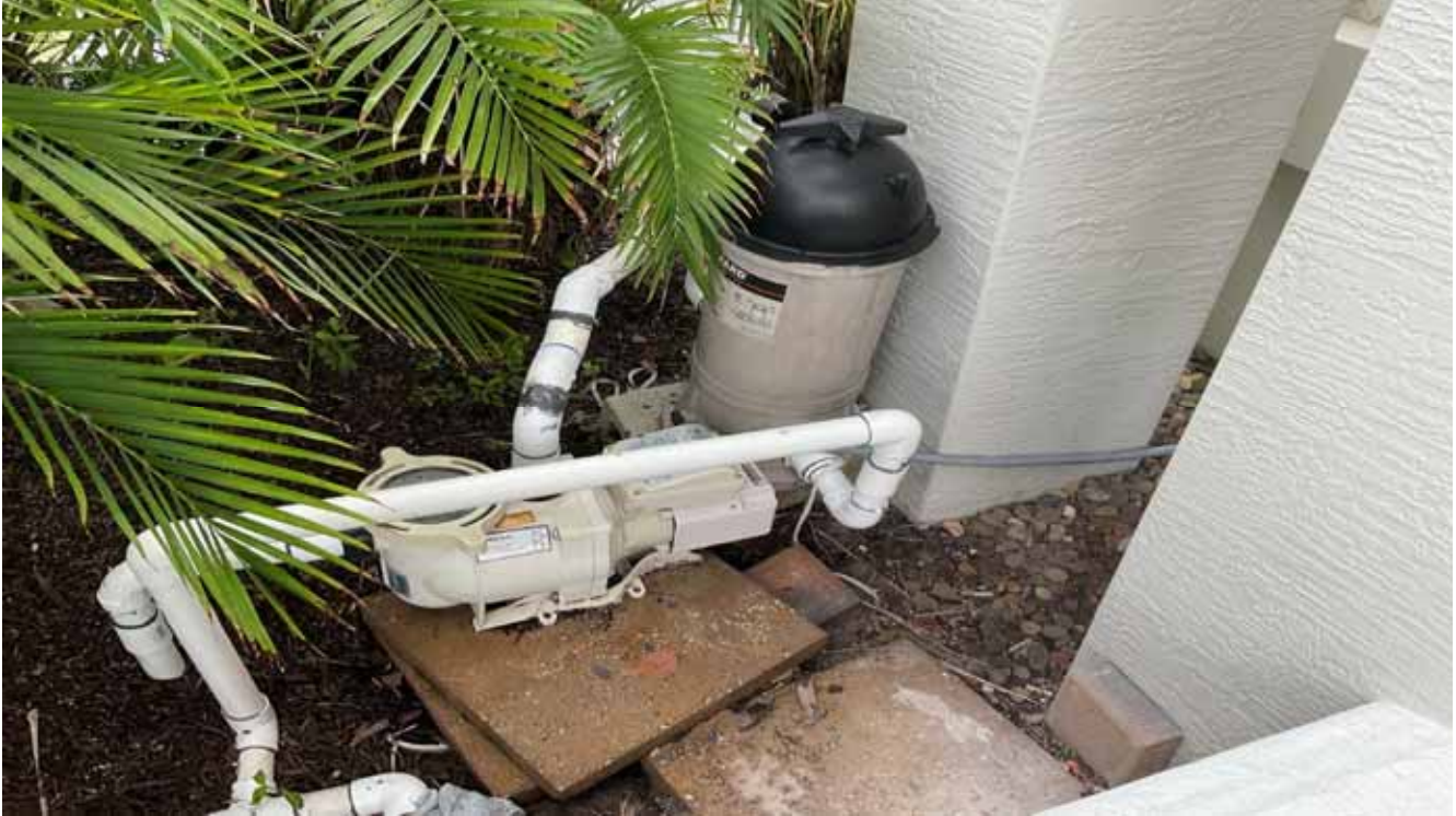
Water Feature Equipment - Clubhouse
