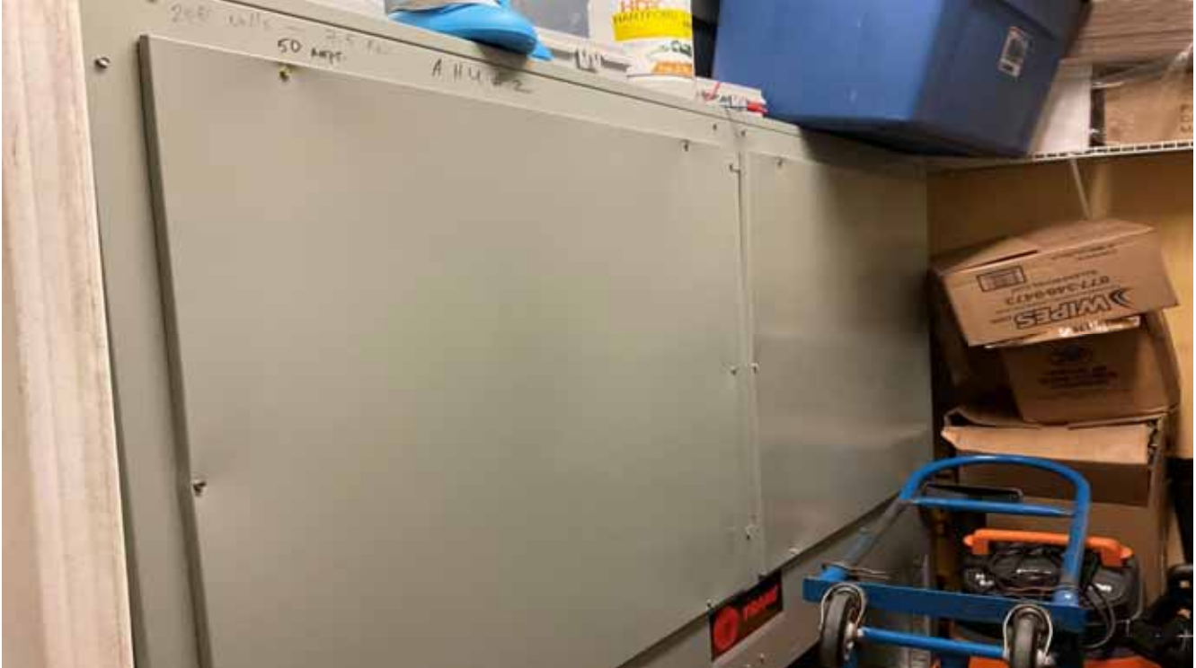
Clubhouse - A/C Unit
