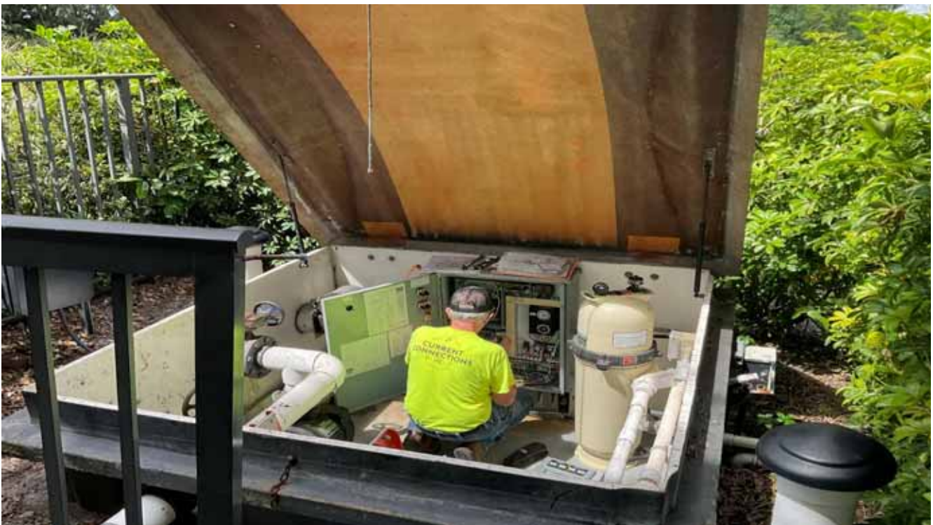
Entry Water Feature Equipment
