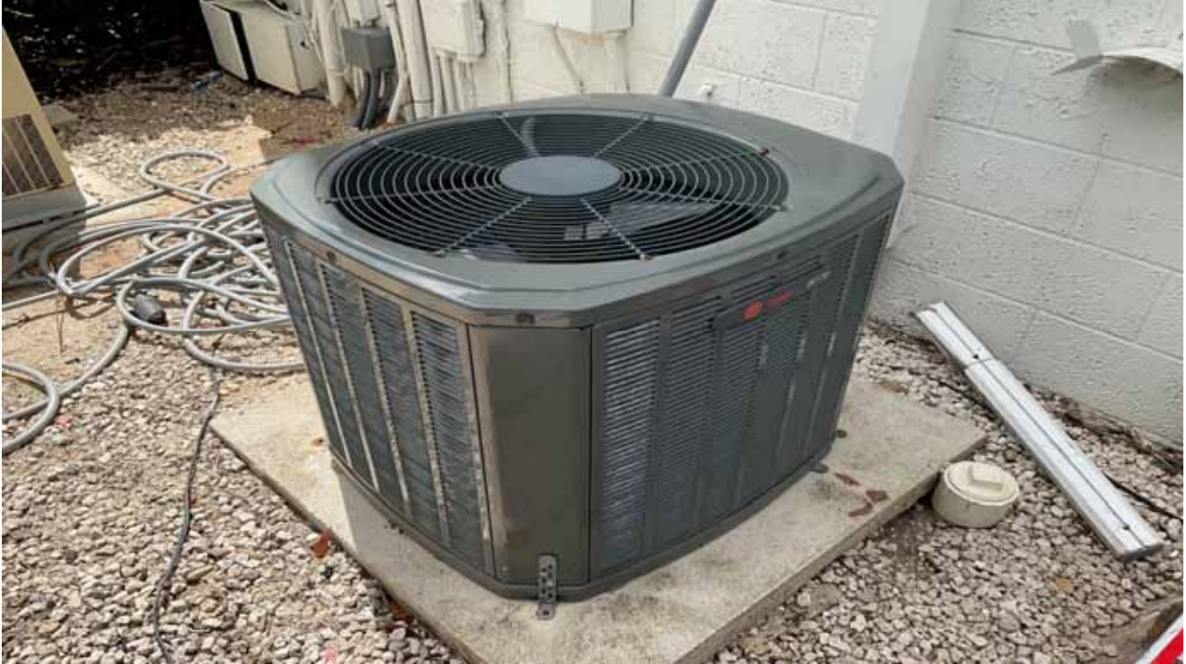
Gatehouse A/C Unit
