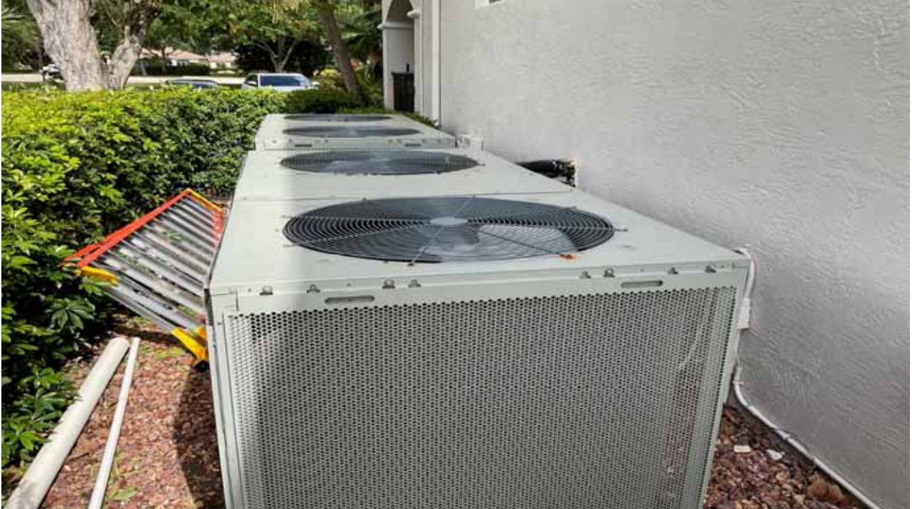
Clubhouse - A/C Units
