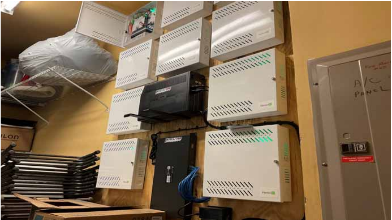
Access Control System Equipment
