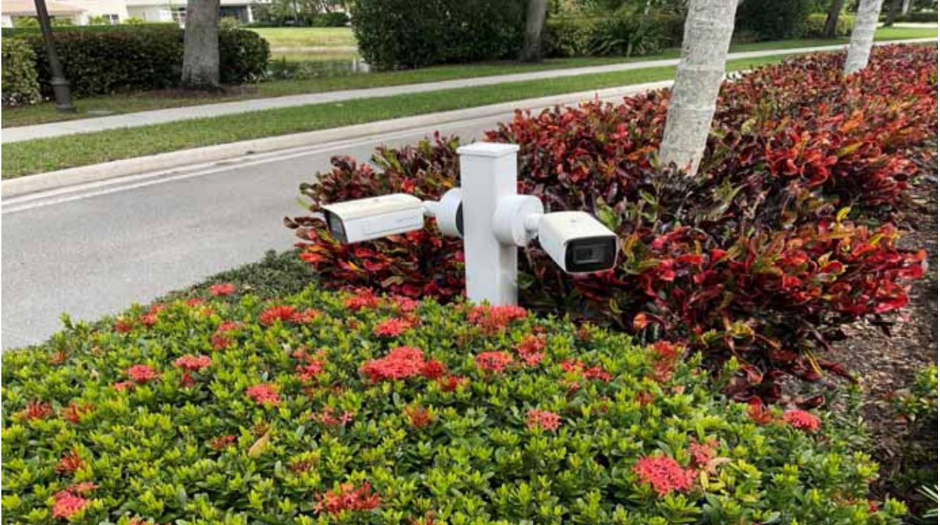
Gatehouse Security Cameras
