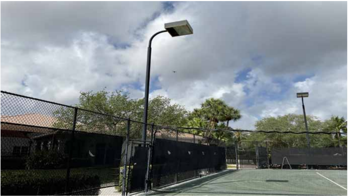
Tennis Court Lighting
