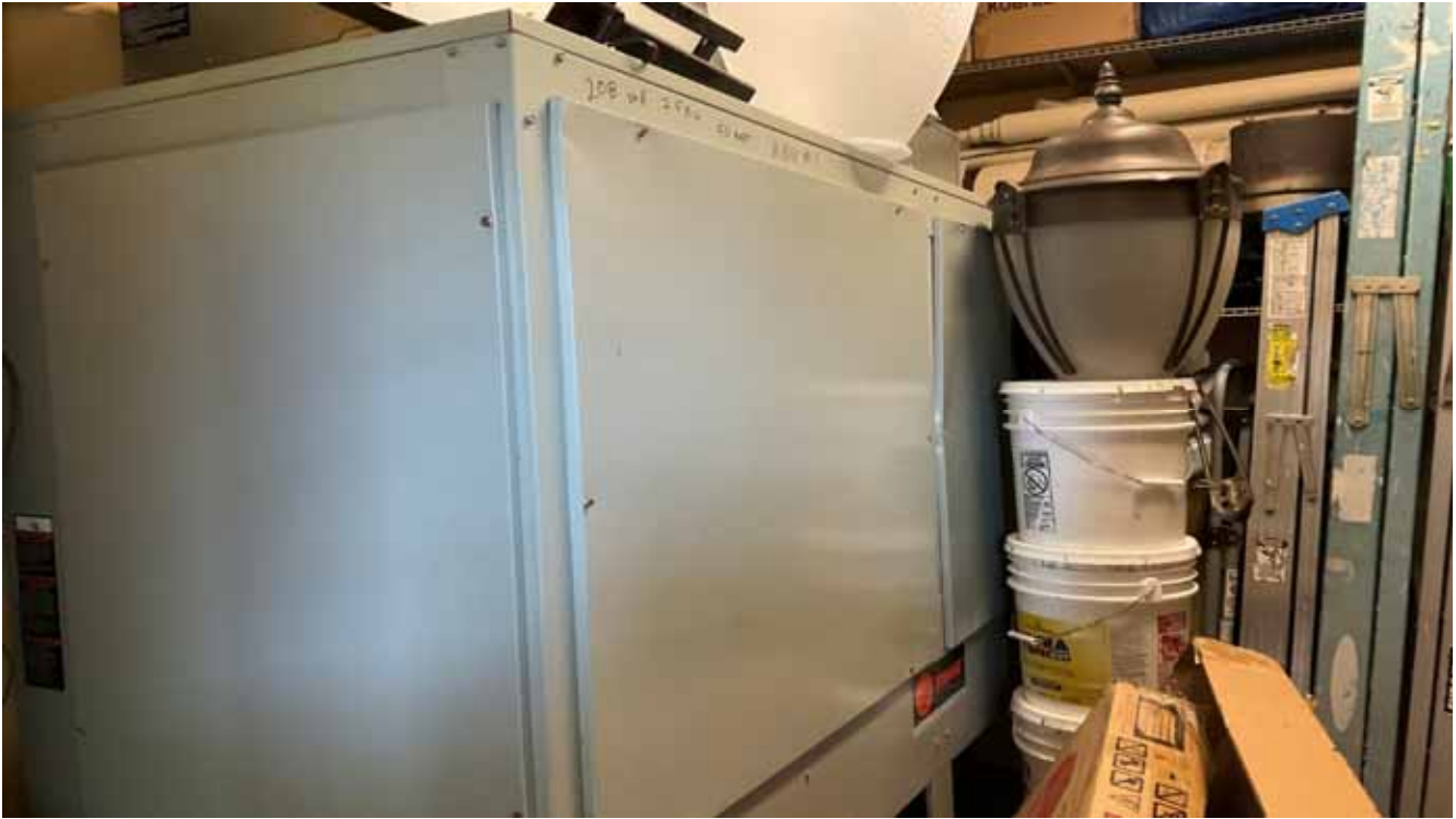
Clubhouse - A/C Unit
