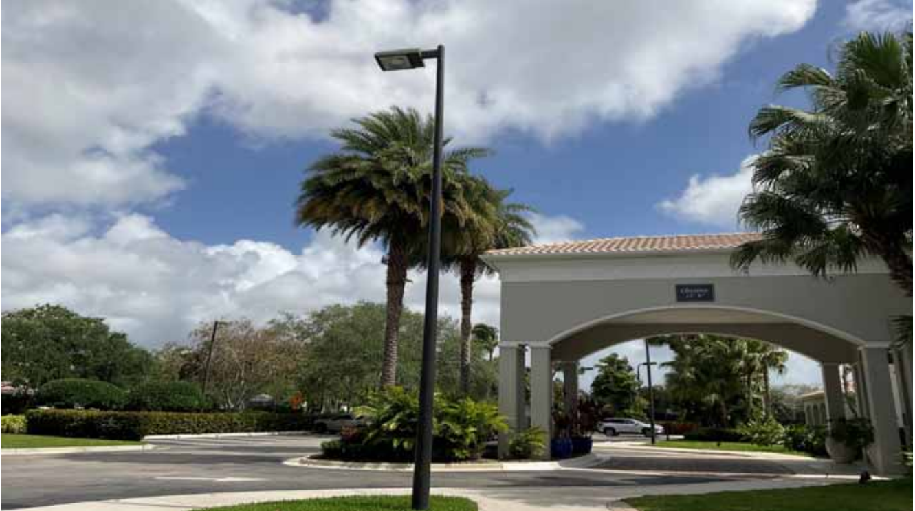
Light Post & Fixture - Parking Lot
