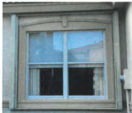
Acceptable: Accordion shutter over top of arched trim at rectangular window opening
