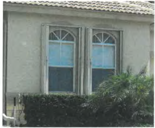
Not acceptable. Top track should be placed above trim or underneath the roof overhang (where it is close)
